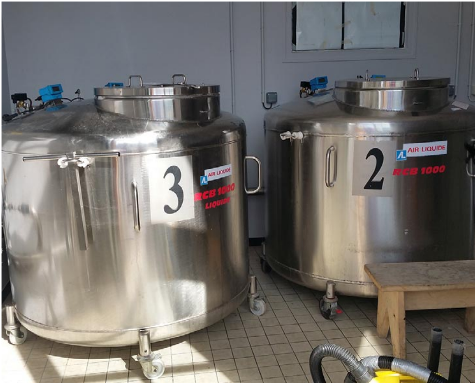
Nitrogen storage tanks
